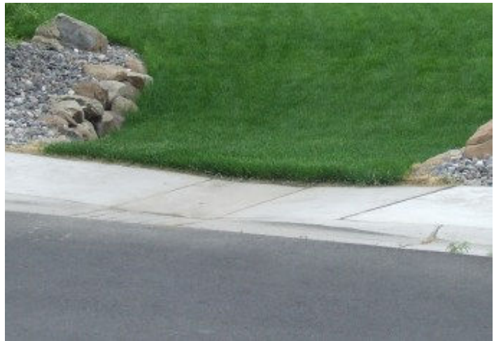
Figure 3 - Construction of this swale did not comply with grading plans. As a result, the depression is not deep enough to effectively infiltrate all stormwater runoff from the street
