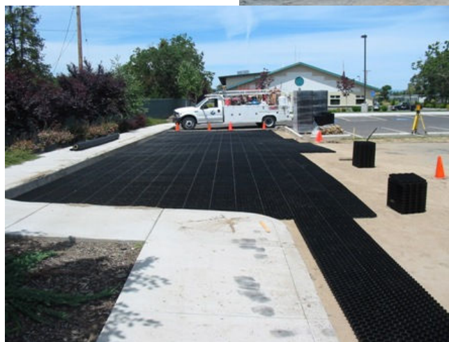
Figures 5 & 6: The layout of the grassy pavers in the parking lot.
